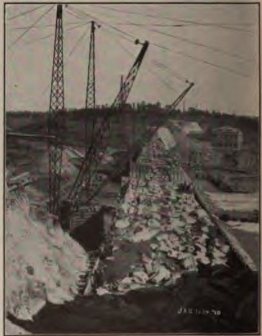
BUILDING THE DAM AT NINETY-NINE ISLANDS, ONE OF THE COM- PANY'S THREE BIG HYDRO-ELECTRIC GENERATING PLANTS
