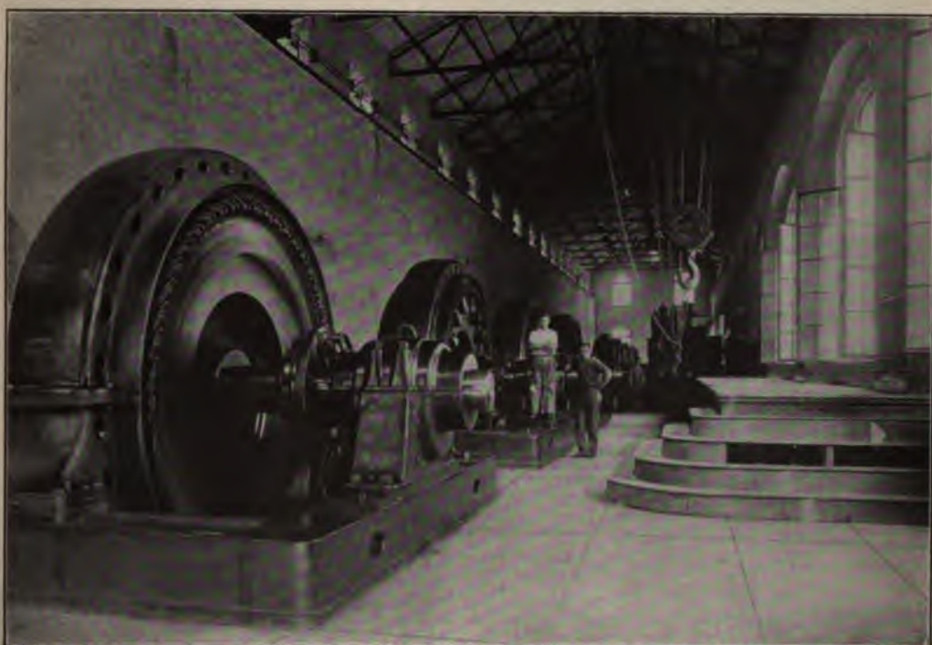
THE GENERATORS AT THE GREAT FALLS STATION PART OF THE SYSTEM WHICH SUPPLIES POWER ALMOST ACROSS TWO STATES
