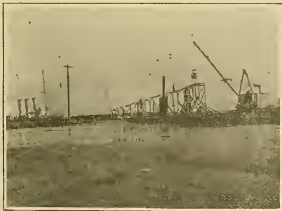
Scene in Third District showing levee construction, mud pumped through elevated sluices.
