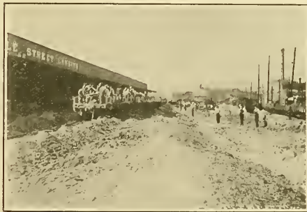
Scene in Third District showing levee construction, material being brought on cars.
