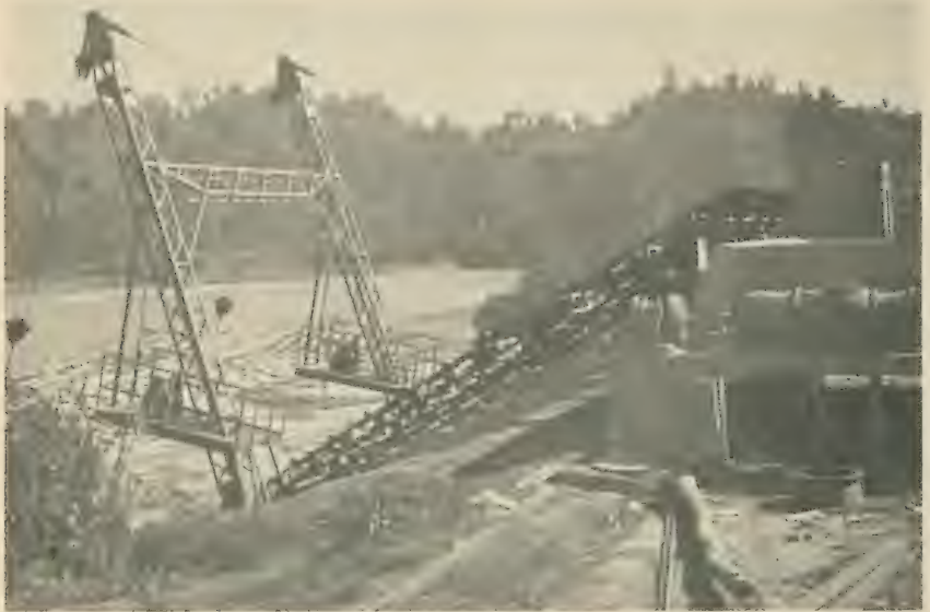
1. At the recently completed Karnaphuli Paper Mill, East Pakistan, bamboo will be used to produce 100 tons of pulp per day. Equipment shown was specially designed to lift rafted bundles of bamboo from the river to the flume, by way of which they will reach the mill.
